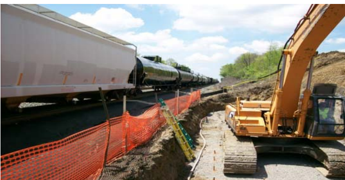
Train at 50 MPH near Quincy foundation.
